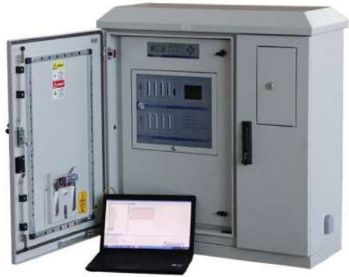
MAESTRO Controller Intersection Controller
